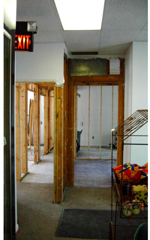
The photo to the right was taken at the top of the entrance stairs looking south towards what would eventually be the entrance to the Grande Parlour. The Grande Parlour was originally five offices. The walls that separated the offices were torn down in 2005 to create one large room— The Grande Parlour.
